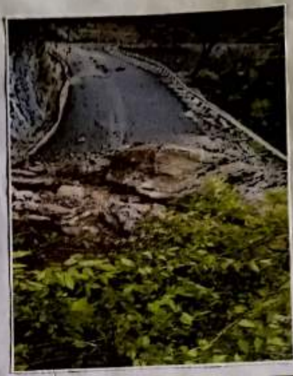
Leaship-Nayabazar road was damaged due to landslides
