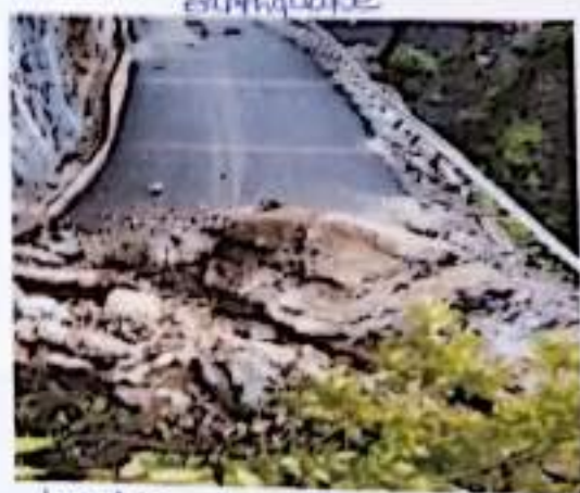
Leqship - Nayabaran road was damaged due to landslide
