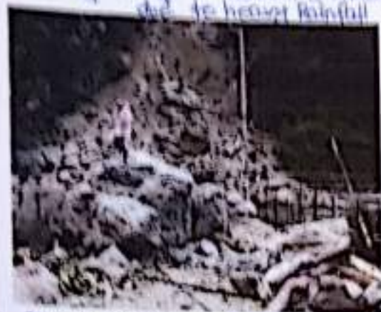
Tangsa Stage - V dam was broken due to landslide
