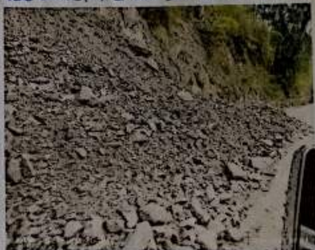
Subsidence of slope
