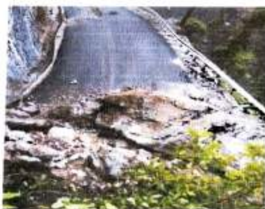
Legship - Nayabazar road was damaged due to landslide
