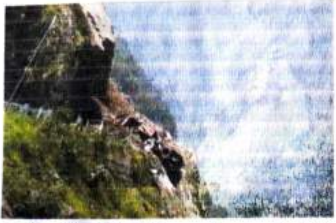
7. Namchi-Rabongla road was closed due to landslide.
