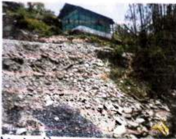
landslide prone area around plain settlement
