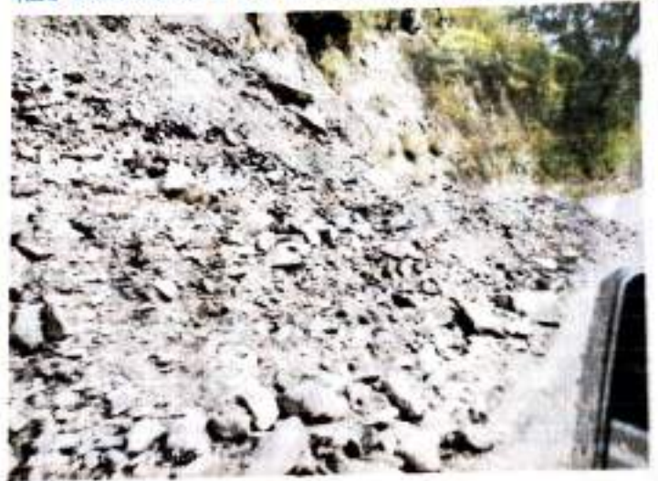
4. Subsidence of slope.
