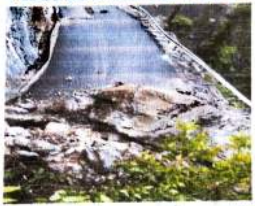
6. Legship-Nayabazar road was damaged due to landslide.
