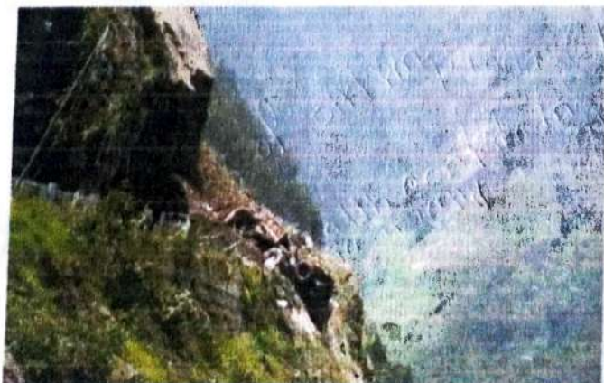
Namchi - Ravangla road was closed due to landslide
