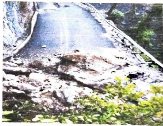
Leogshup - Mayajaborar road was damaged due to landslides
