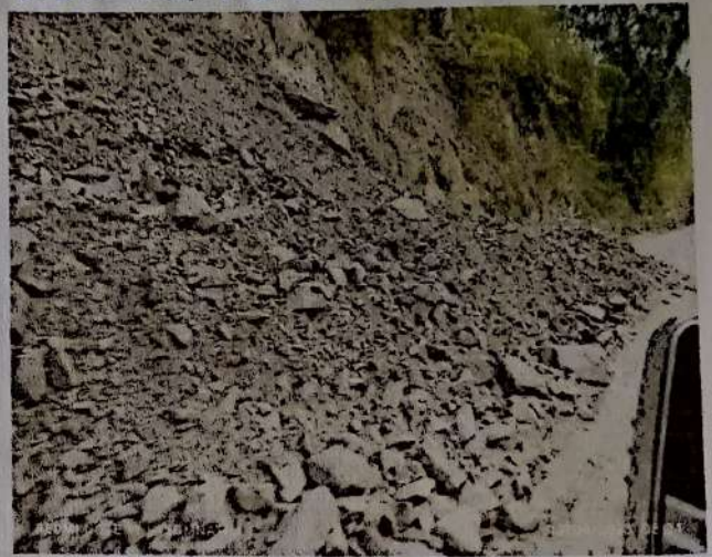
Subsidence of slope
