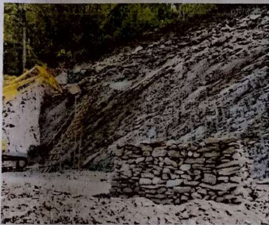
Rock slope netting
