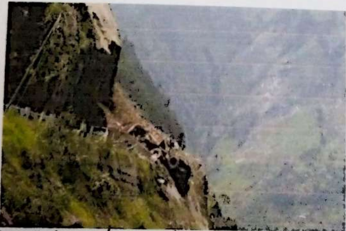
Nomechi Rabangla Road was closed due to landslide.
