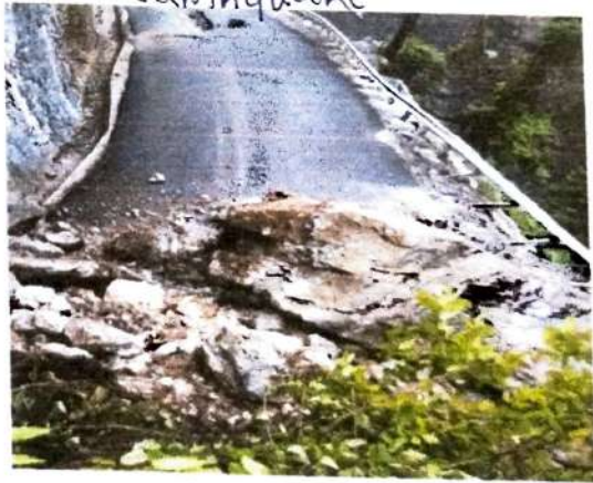
6. Legship Nayabazan road was damaged due to landslide
