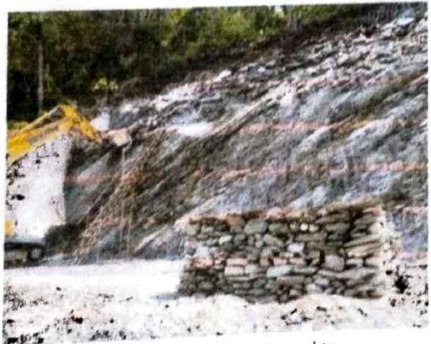
5. Rock slope Netting
