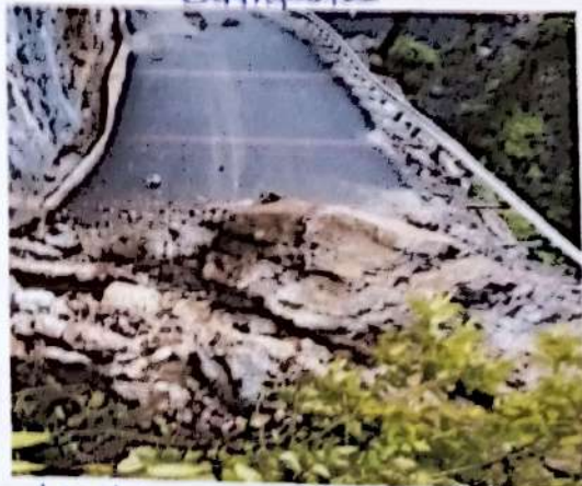
Legship - Nayabaran road was damaged due to landslide
