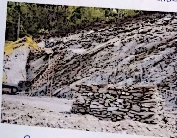
Rock Slope Netting
