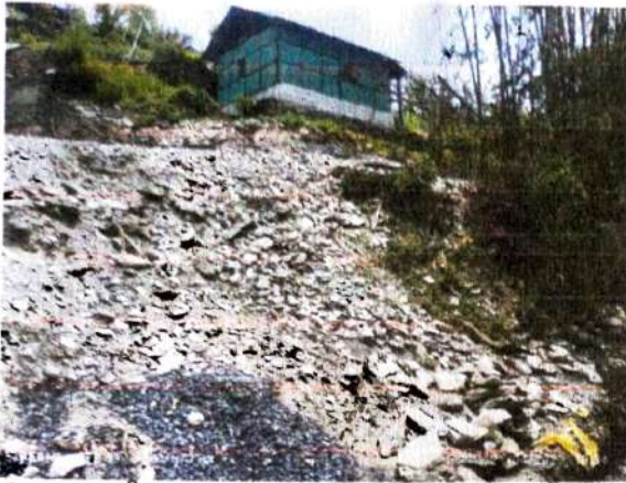
Landslide prone area Unplanned settlement
