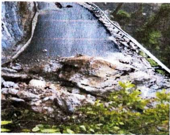
Legship - Mayabazar road was damaged due to landslides
