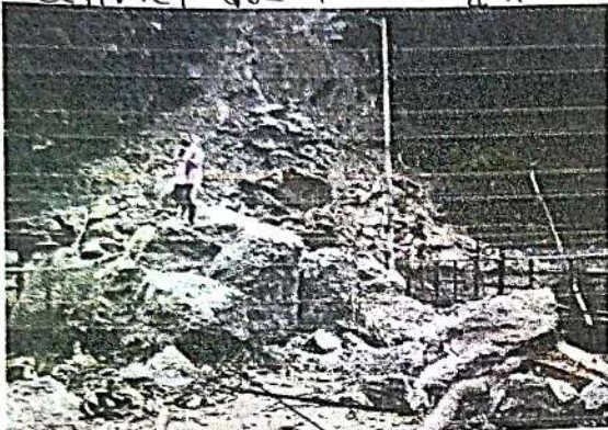
Teesta stages - V dam was broken due to landslide
