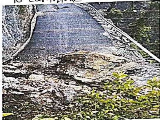
Legship - nayabazar road was damaged due to landslide
