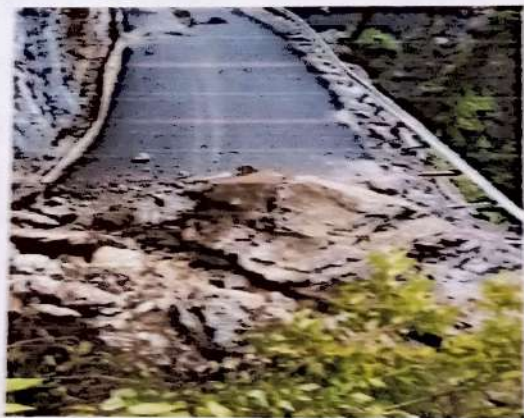
Legship - Nayabozan road was damaged due to landslide
