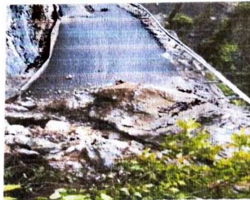
6. Legship-Nayabazar road was damaged due to landslide.
